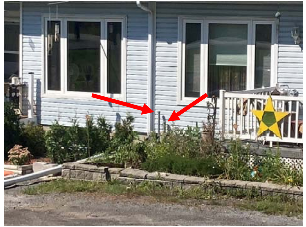
Photo 10. View of the vent pipe (see left arrow) and fill pipe (see right arrow) observed on the neighbouring property to the southeast of the Phase One Property at 1201 Old Montreal Road.
