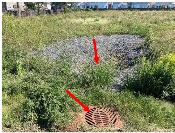
Photo 5. View of the two catch basins (see arrows) observed on the northwest portion of the Phase One Property.
