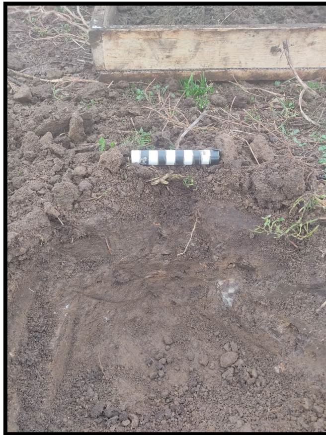
Figure 6: Typical test pit excavation in progress complicated by larger limestone cobbles in walls (PA1214-D32).
