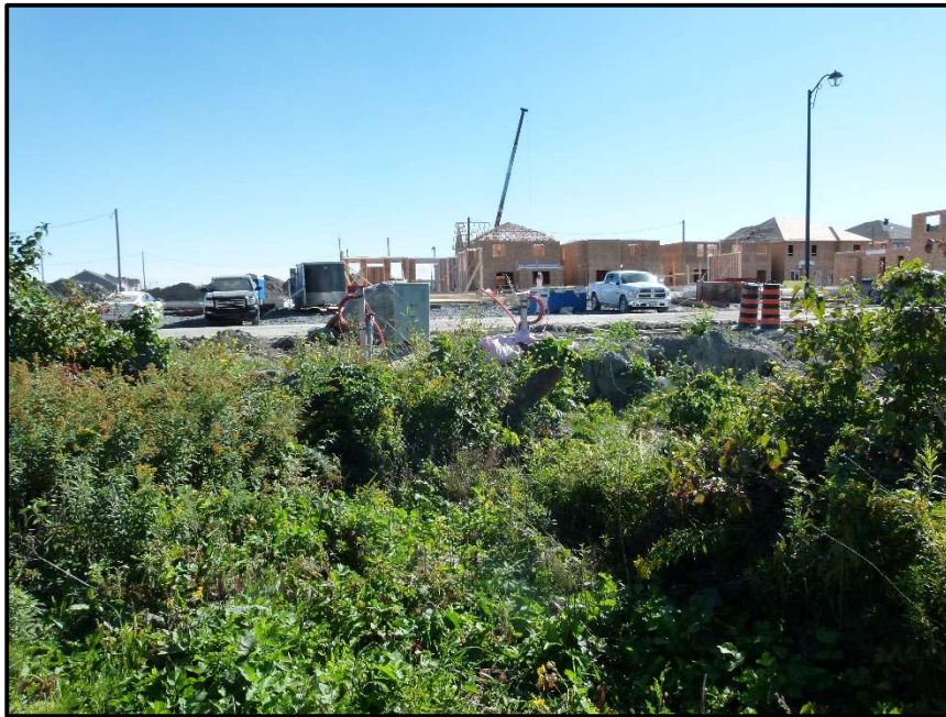
Photograph 16: Looking south at the adjacent residential subdivision (under construction). The area shown historically included the upstream portion of Drainage Feature C (September 17 th , 2020).
