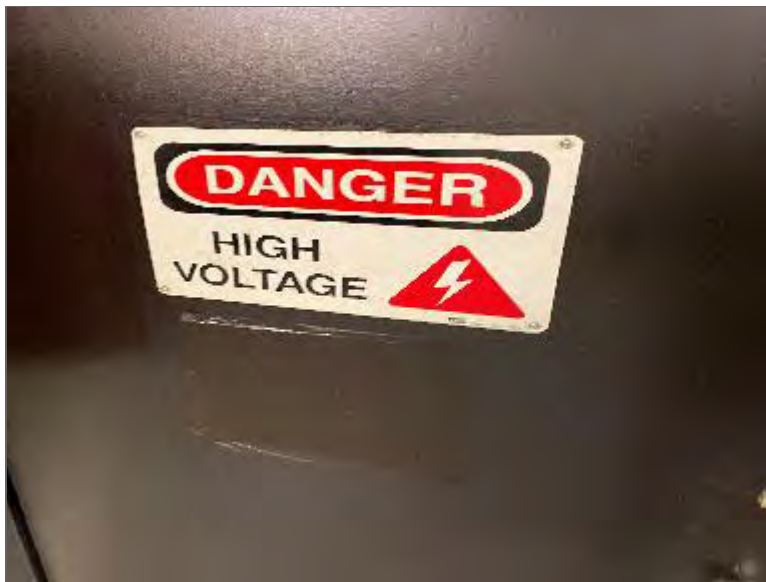
Photo 6 – Hydro vault (PCA) located in the southwest portion of Site Building A.
