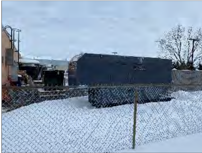
Photo 11 – Emergency generator (with associated diesel AST, a PCA) located at 2060 Walkley Road.
