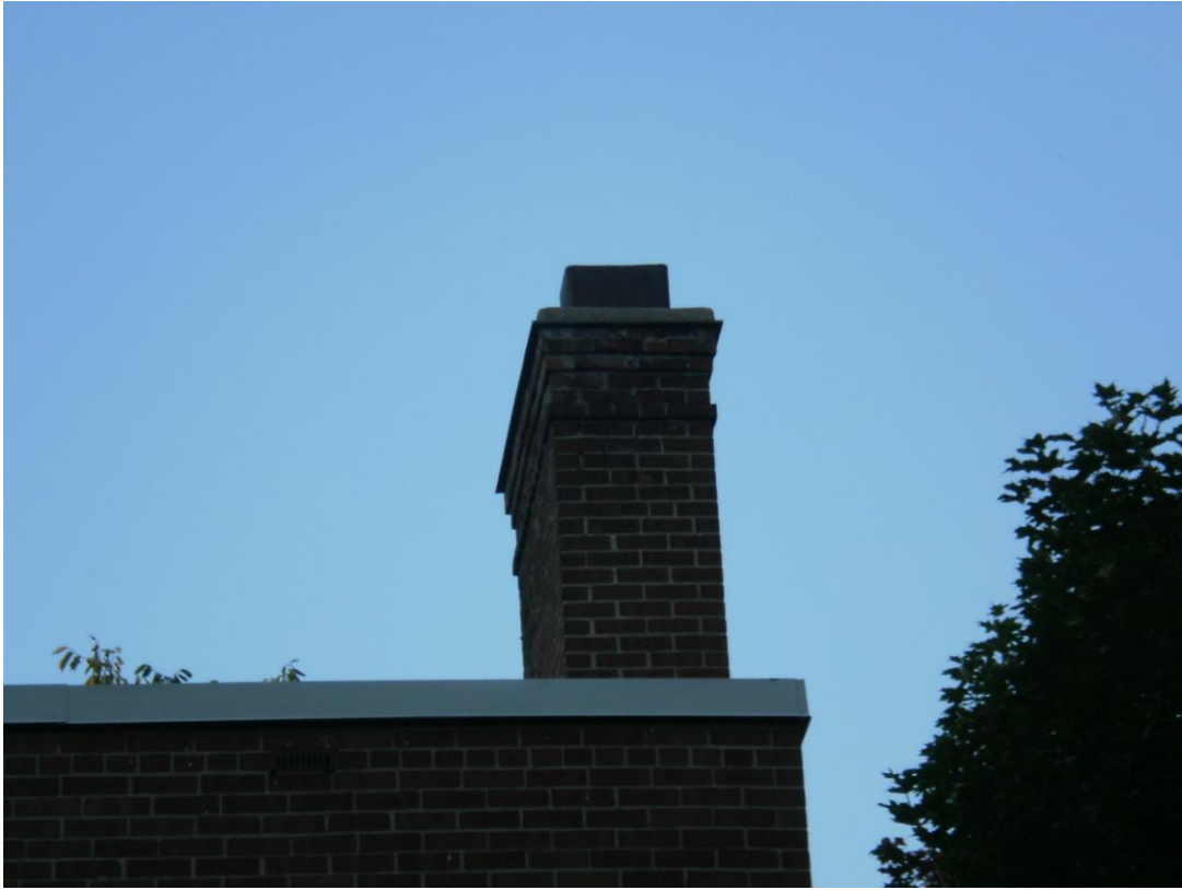
Photo 1 – Open brick chimney on the top of the building at 231 Cobourg Street
