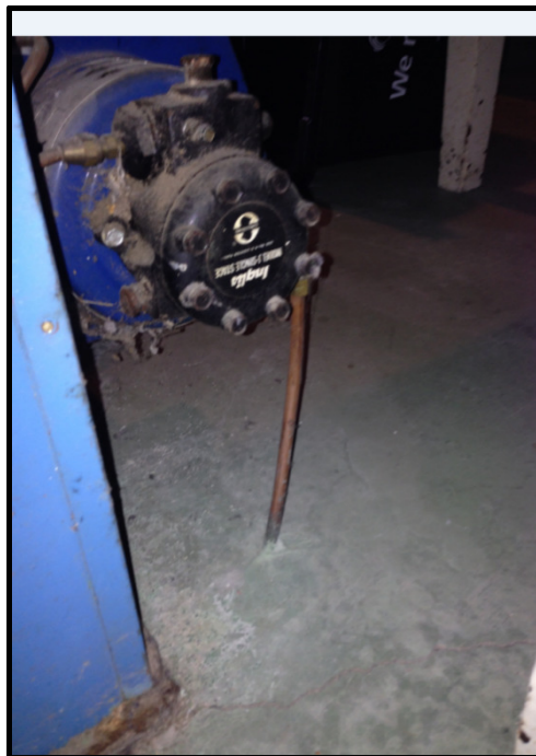
Photograph 14: Photograph illustrates copper oil line at 534 Edison Avenue, exiting the concrete floor slab in the vicinity of the furnace.
