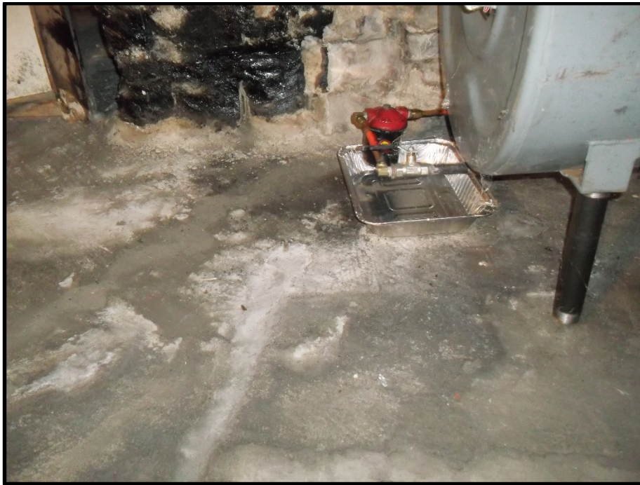
Photograph 11: Photograph illustrates portion of AST in the basement of 530 Edison Avenue, as well as some staining on the concrete floor slab and the location of the partially buried former oil line.
