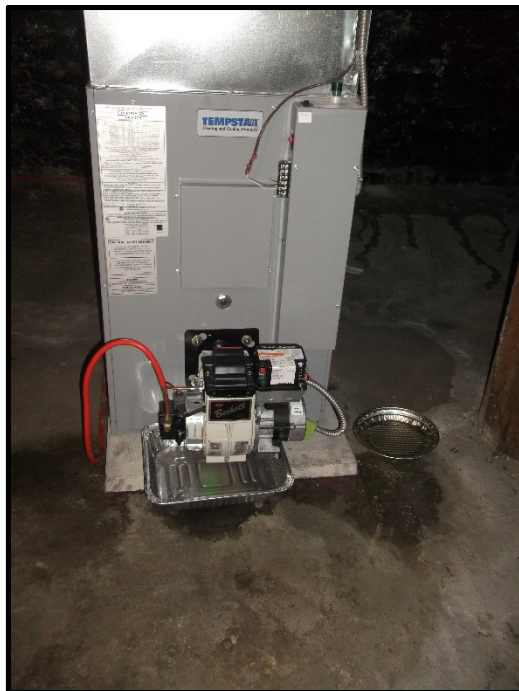
Photograph 12: Photograph illustrates the furnace at 530 Edison Avenue and staining on the surrounding concrete floor slab.
