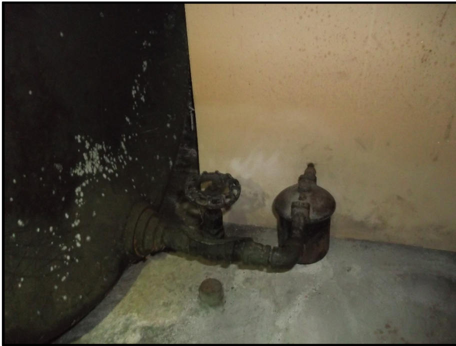
Photograph 13: Photograph illustrates a portion of AST at 534 Edison Avenue, a 2.5 cm capped pipe in the concrete floor and the copper line leading behind the drywall.
