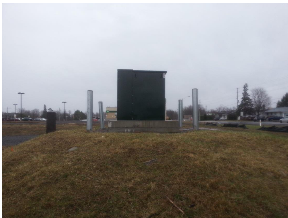
Photograph 8: Off-Site pad mounted transformer #1 (grocery store property, near Shea Road).
