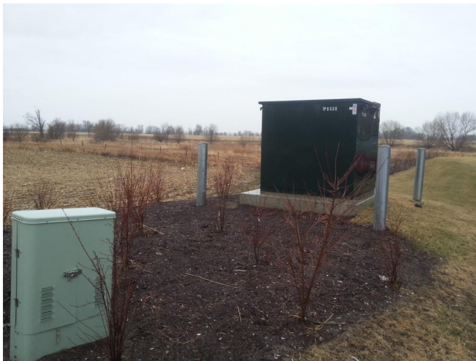
Photograph 11: Pad mounted transformer #2 (located southwest of the grocery store building).
