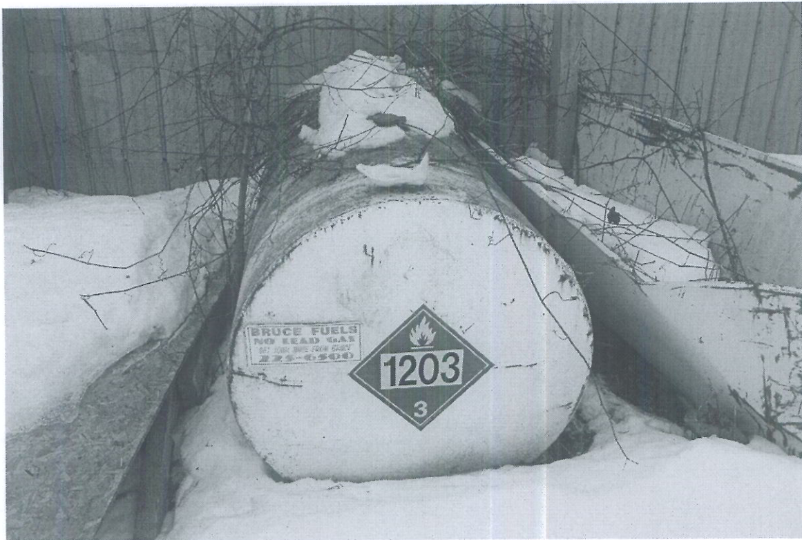
Above Ground Fuel Storage Tank located on North Side of Storage Building
