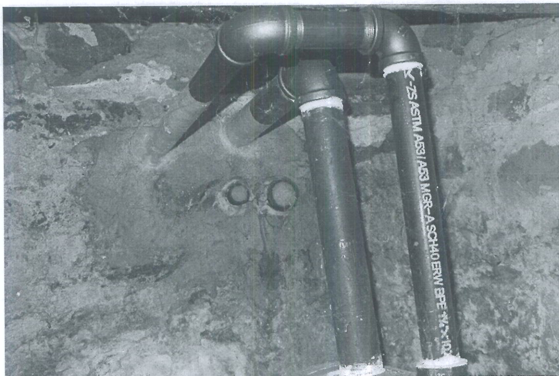
Former and Newly Installed Fill Pipes for Fuel Oil Storage Tank in Basement
