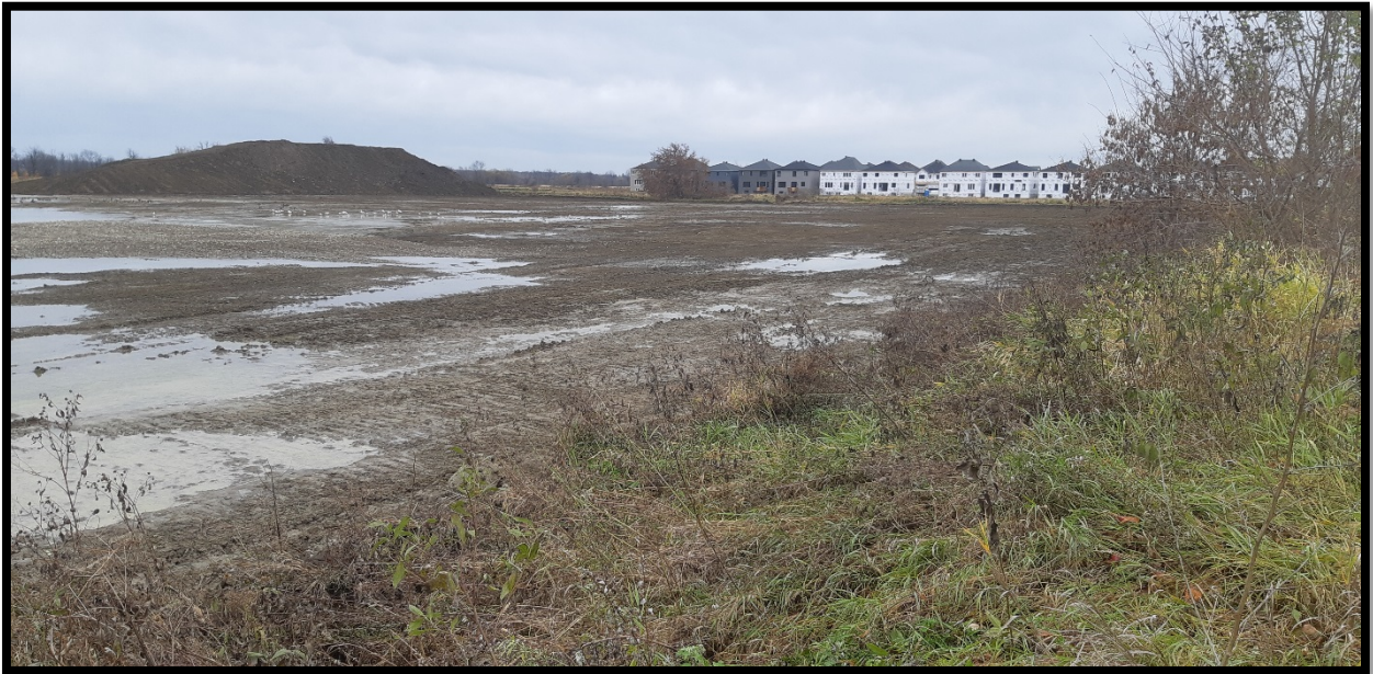
Figure 4: Western most portion of study area, showing stripping and dirt pile. (PA1138-D05)
