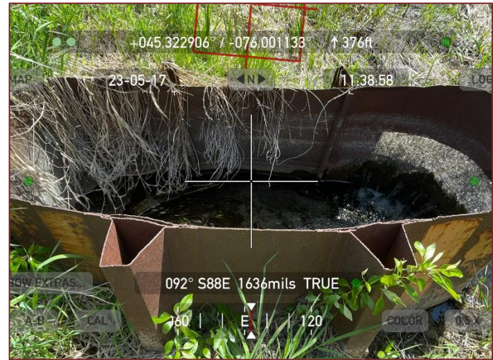
Site Photograph 6: The vertical drain on-site.
