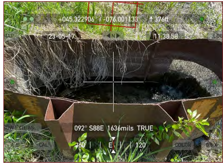
Site Photograph 6: The vertical drain on-site.
