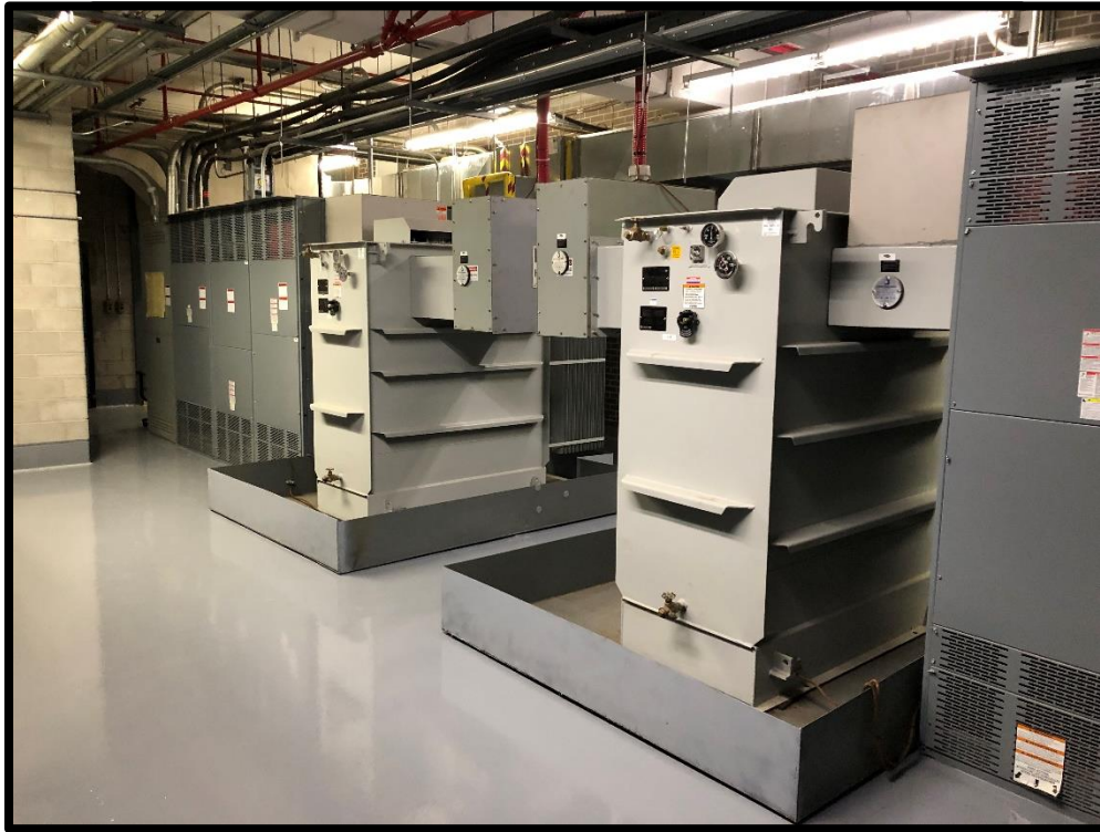
Photograph 7: View of the two liquid phase transformers in the basement of the Brooke Claxton building.
