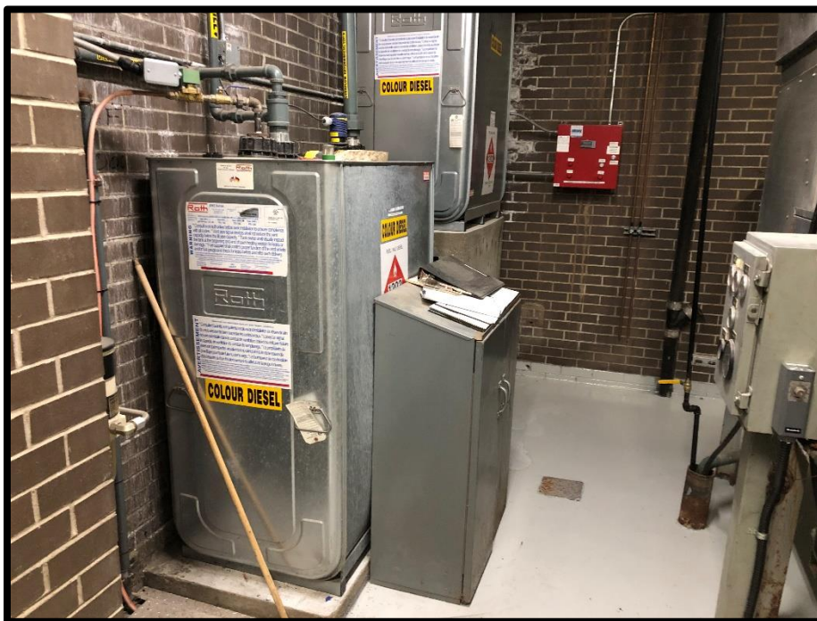
Photograph 5: View of the two 1,000 L ASTs in the basement of the Brooke Claxton building.
