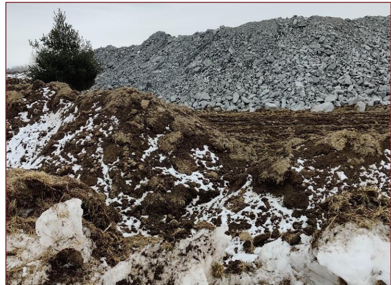
Site Photograph 8 – Crushed rock and tilled native material on the southwest portion of the Site.
