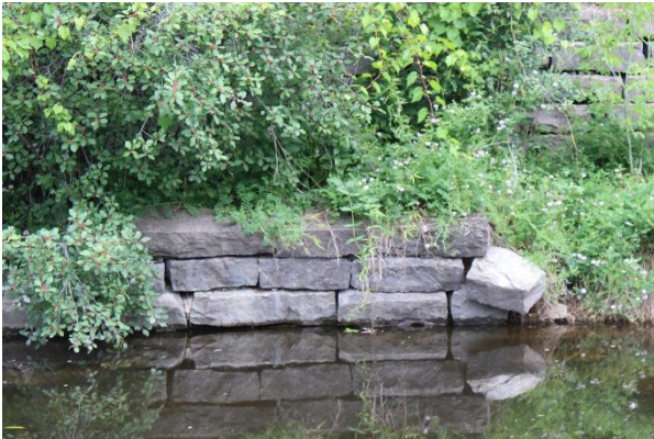
Photo 4.19: Damage to stone wall
