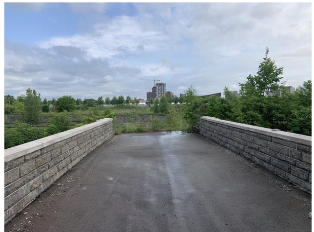
Photo 12: Aqueduct deck surface over Fleet Street Tailrace in OA (Open Water), facing north.
