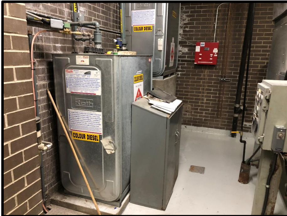
Photograph 5: View of the two 1,000 L ASTs in the basement of the Brooke Claxton building.
