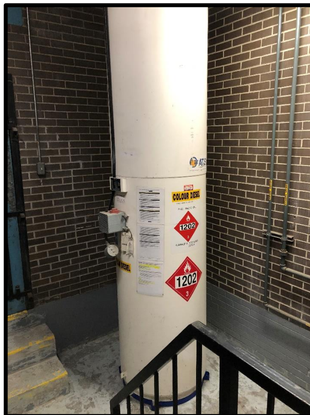
Photograph 6: View of the 2,275 L AST in the basement of the Brooke Claxton building.
