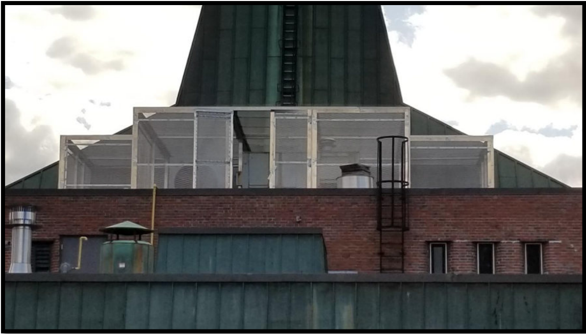
Photograph 4: View of the rear of Building A of the Site, facing south. Rooftop mechanical equipment is present on top of the building.
