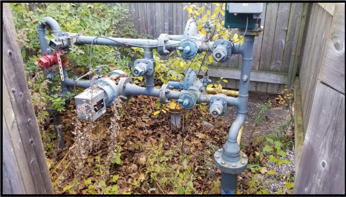
Photograph 7: Natural gas enclosure, observed between Buildings B and M. Site utilities are present underground, throughout the complex.
