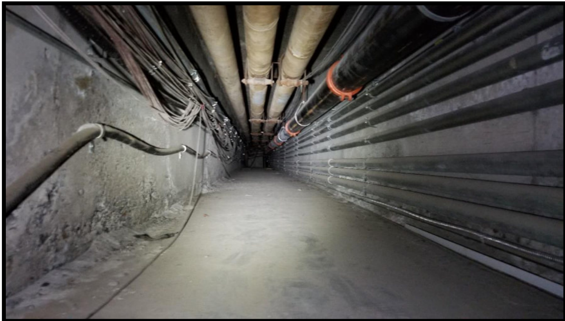
Photograph 10: View of a utility tunnel between two buildings within the complex (July 2019).
