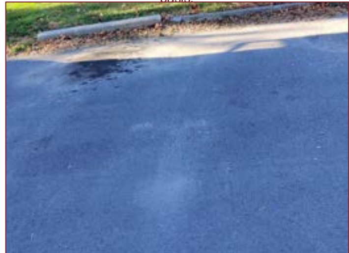
Photograph I12 – Oil staining (appeared to be surficial) in one of the asphalt parking lot at the Site.
