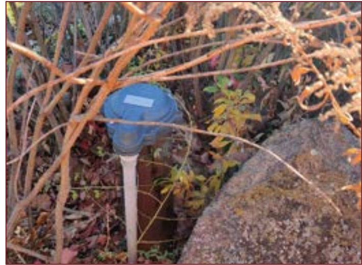
Photograph I2- On-Site water well for the Site.
