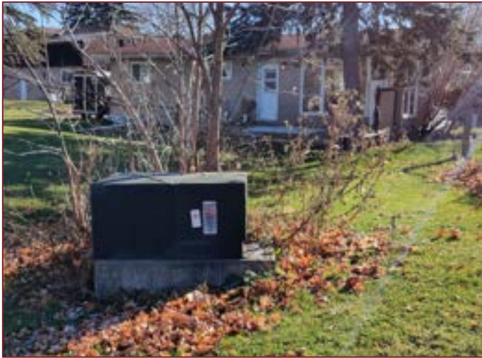
Photograph I9 – Transformer located on the Site closer to the northern boundary.
