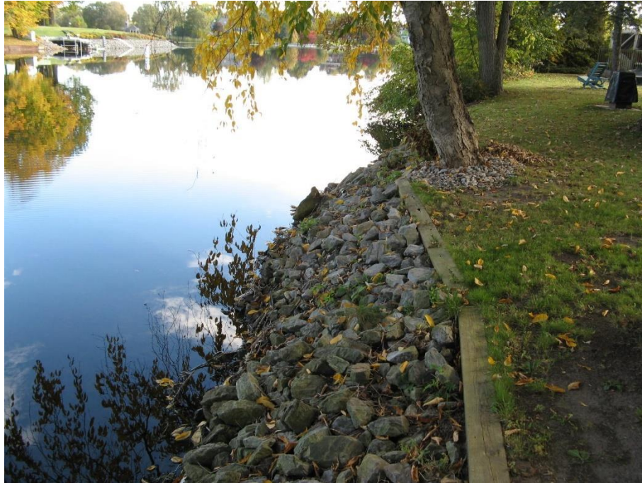
Photo 9 – Typical hardened shoreline conditions with rock protection, good tree cover, and mowed landscape. View looking east along north edge of site
