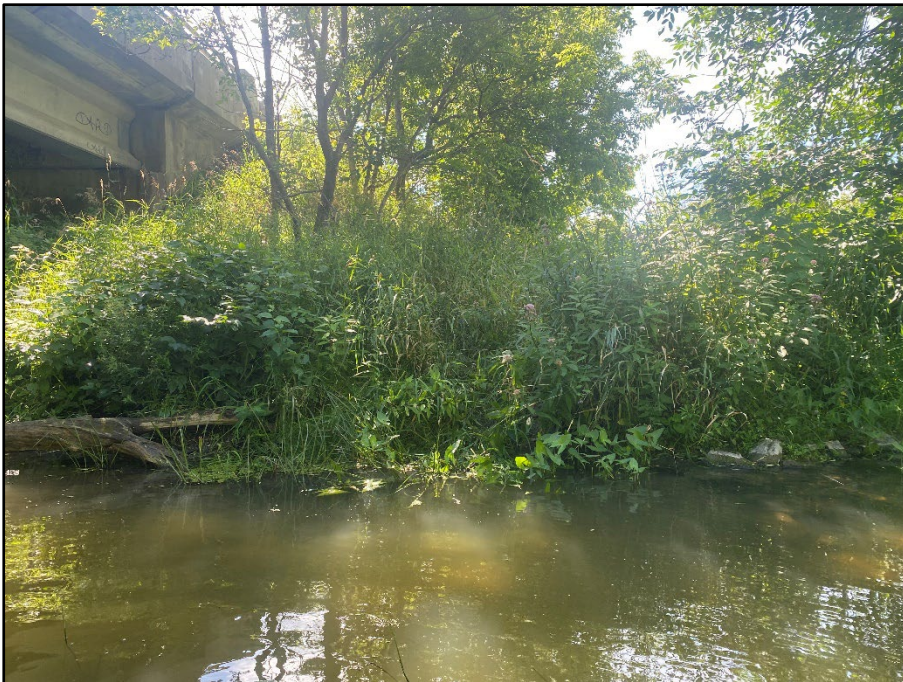
10. Mud Creek – Facing parallel to Rideau Valley Drive N, inlet location from the Oxbow feature into Mud Creek with an approximate 1 – 1.5 m elevation change
