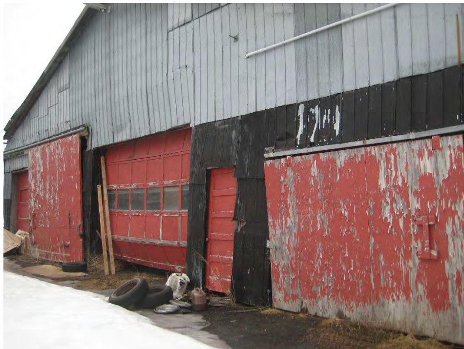
Photograph 8: View of the equipment storage shed located on the Site which was not accessible at the time of the Site visit.
