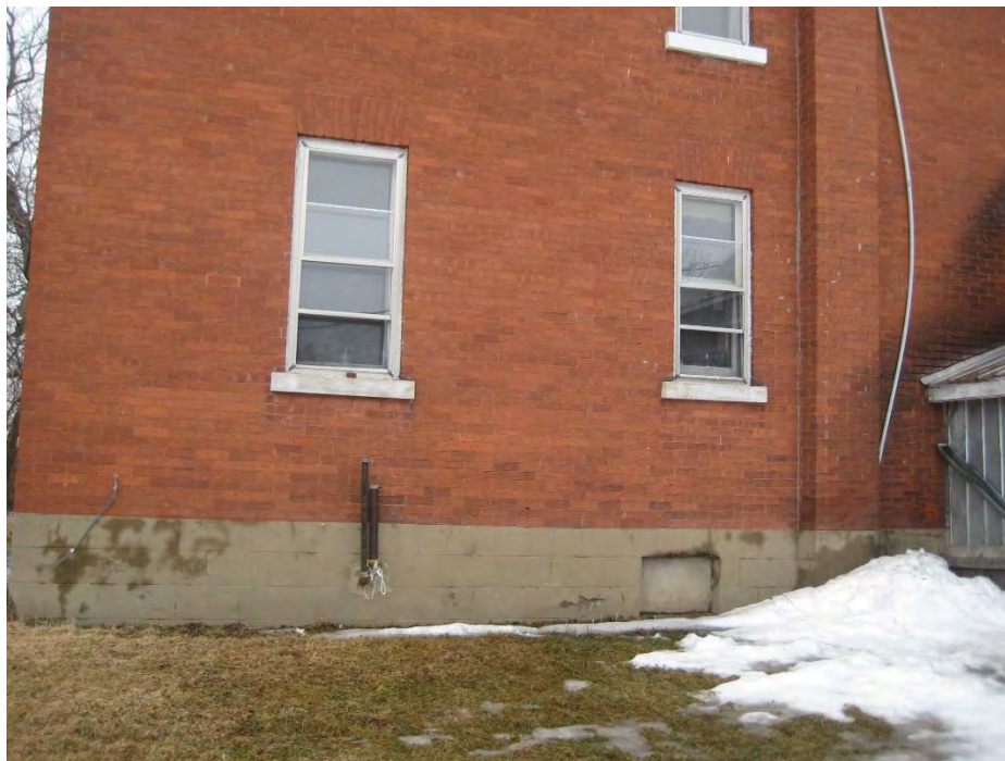
Photograph 10: View of fill and vent pipes on the west wall of the house that are most likely associated with a heating oil aboveground storage tank (AST) located in the basement of the house (not accessible at the time of the Site visit).
