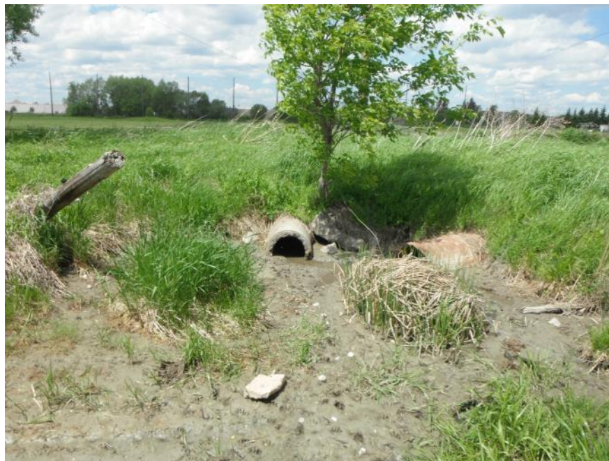
Photo 1 Looking upstream at downstream end of the piped section of the Burnett Municipal Drain (May 21, 2015)
