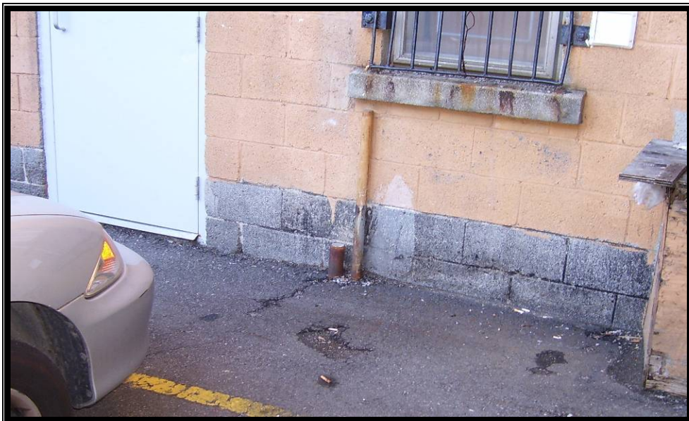
Photograph 4 – Evidence of an abandoned underground storage tank (“UST”), observed just northwest of the Site.
