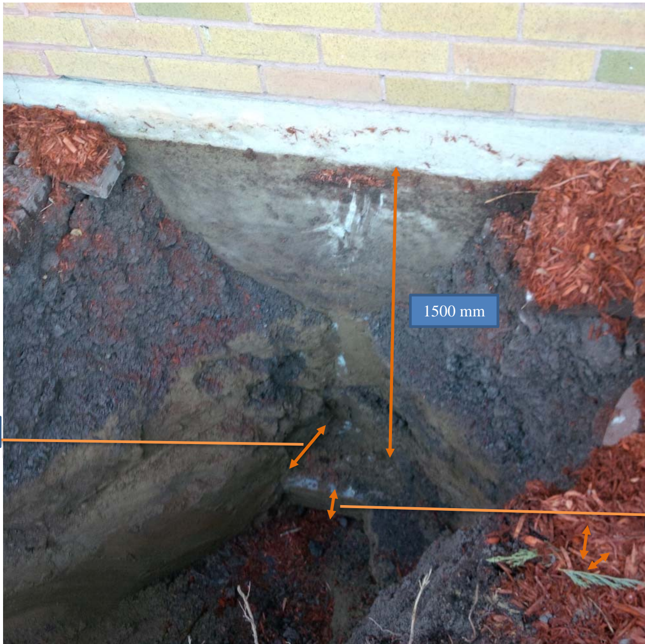
Photo No. B4: Test Pit No. 4- Strip Footing at a depth 1.5 m, Elevation: Founding Material: Silty Sand
