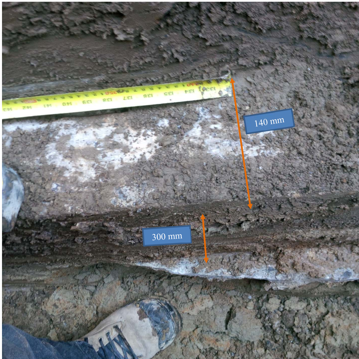
Photo B1: Strip Footing at Test Pit 1 – USF at 1.2 m below Grade – Elevation: Founding Material: Silty Sand
