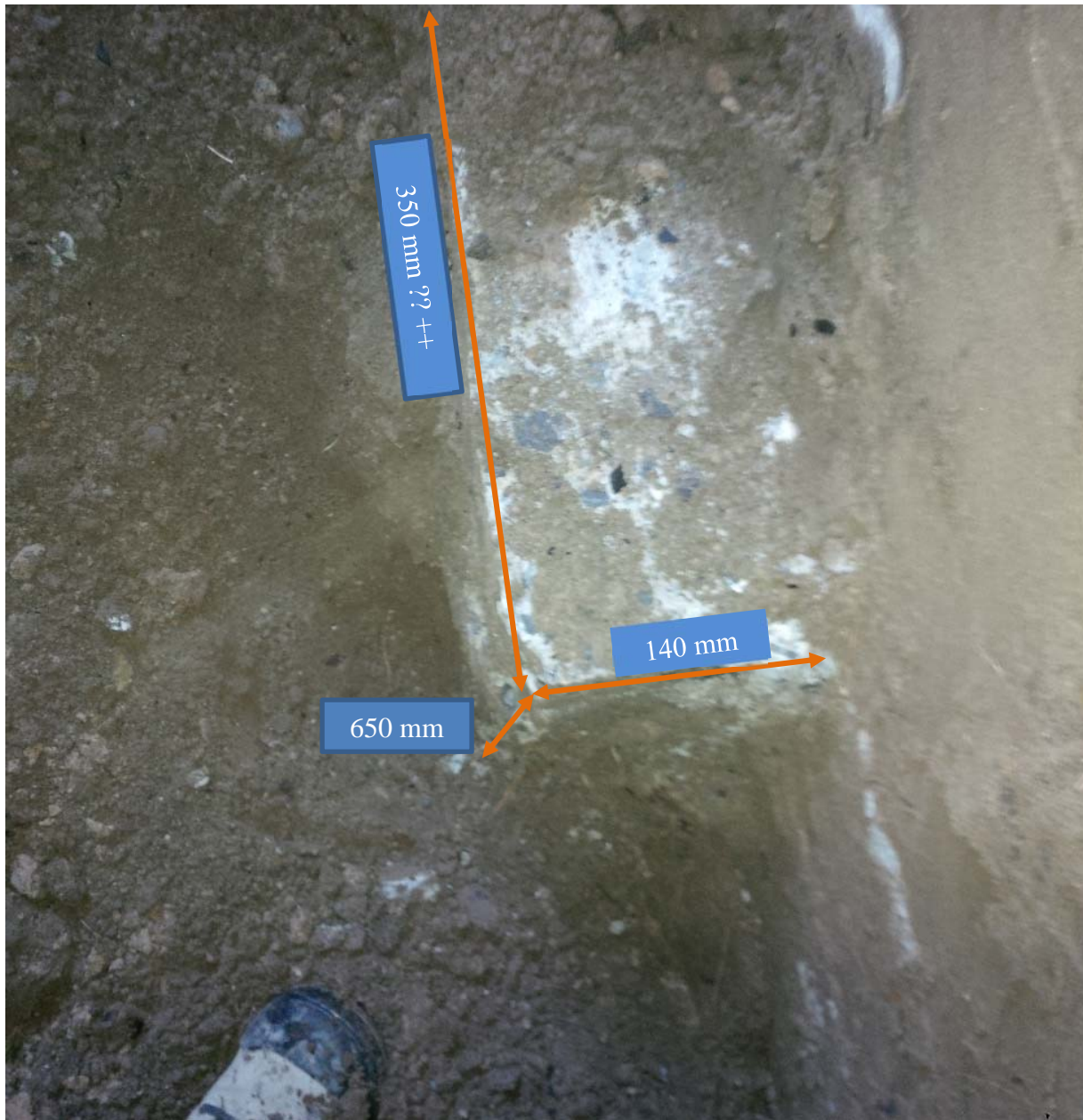
Photo No. B3: Test Pit No. 3- Spread Footing at a depth 2.2 m, i.e. Elevation: xx m (Partial length of Footing was exposed as shown)- Founding Material: Glacial Till
