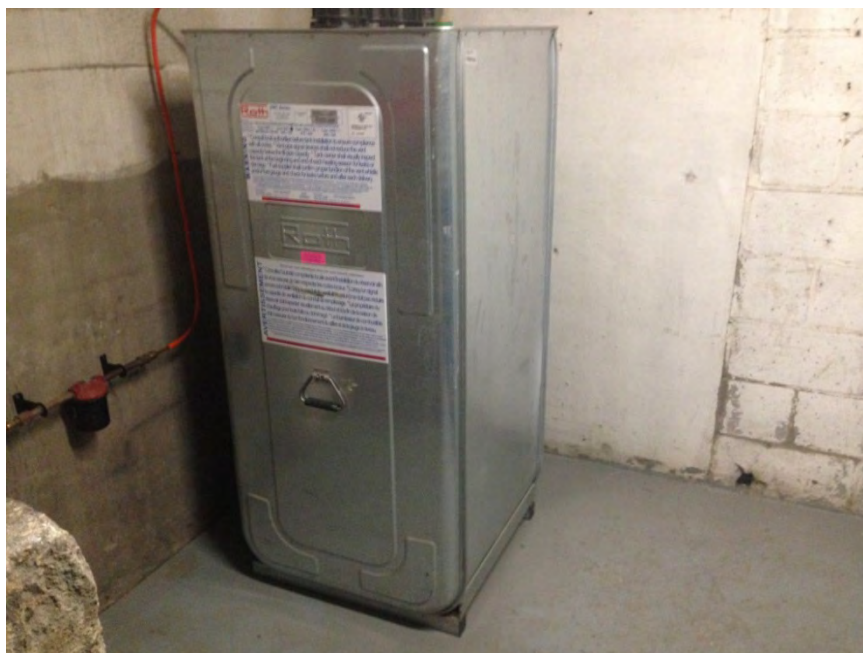
Photograph No. 4 Diesel tank associated with the generator
