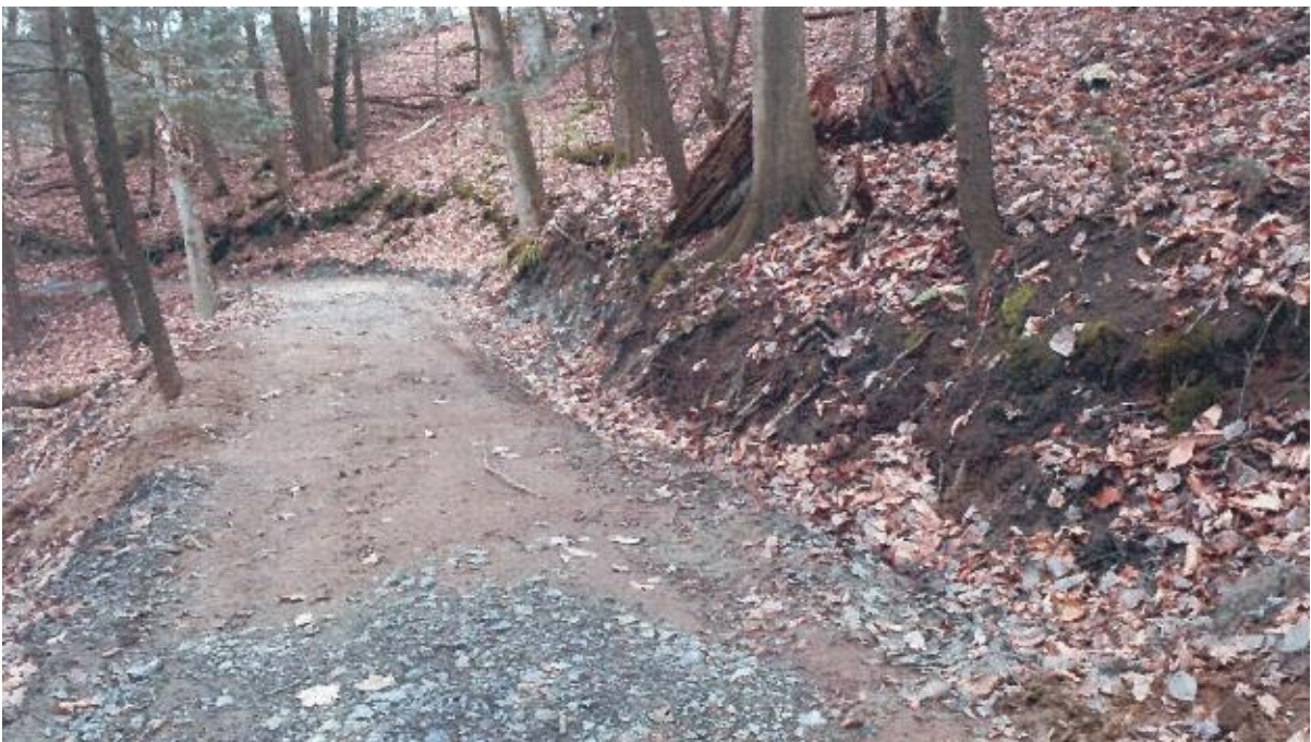
Photo No. 8 – Erosion of cut uphill of pathway. Cut approximately 42 m long x 0.5 m to 1.3 m high.
