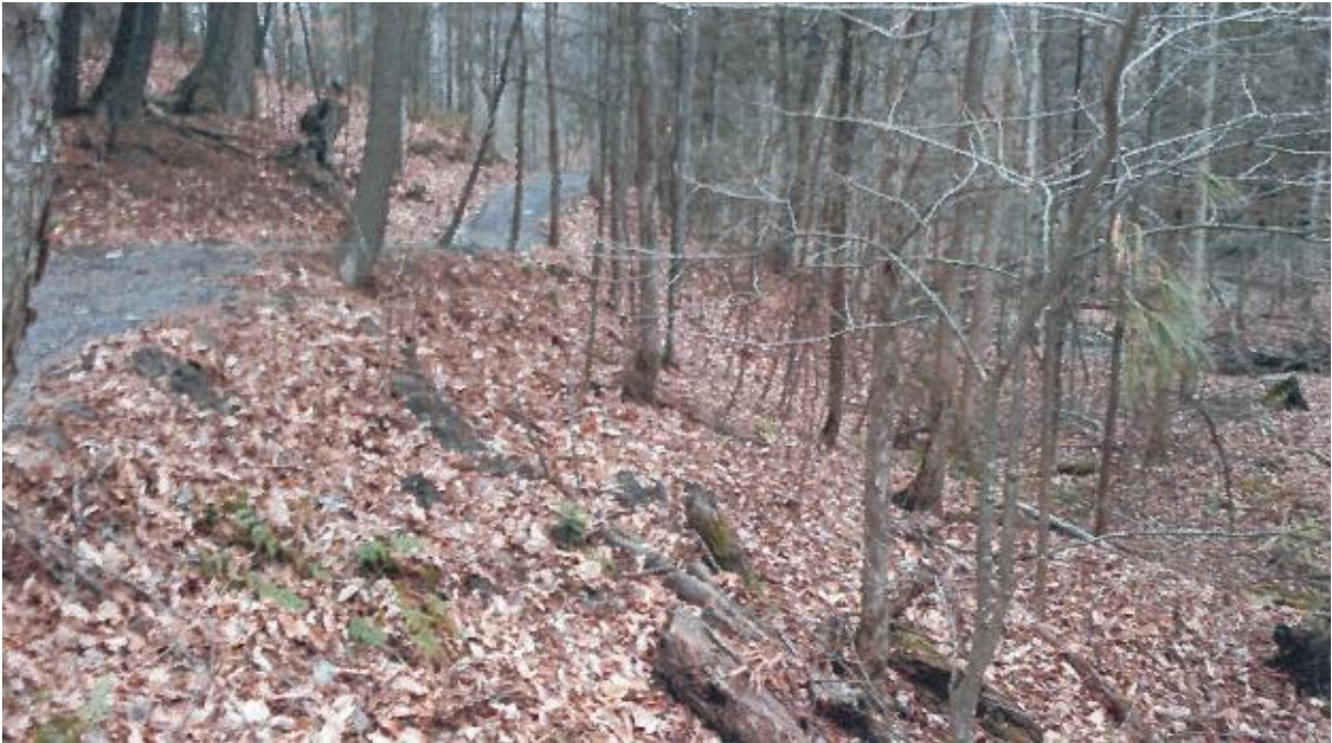
Photo No. 22 – Erosion below pathway. Cut approximately 30 m long x 0.5 to 2 m high.
