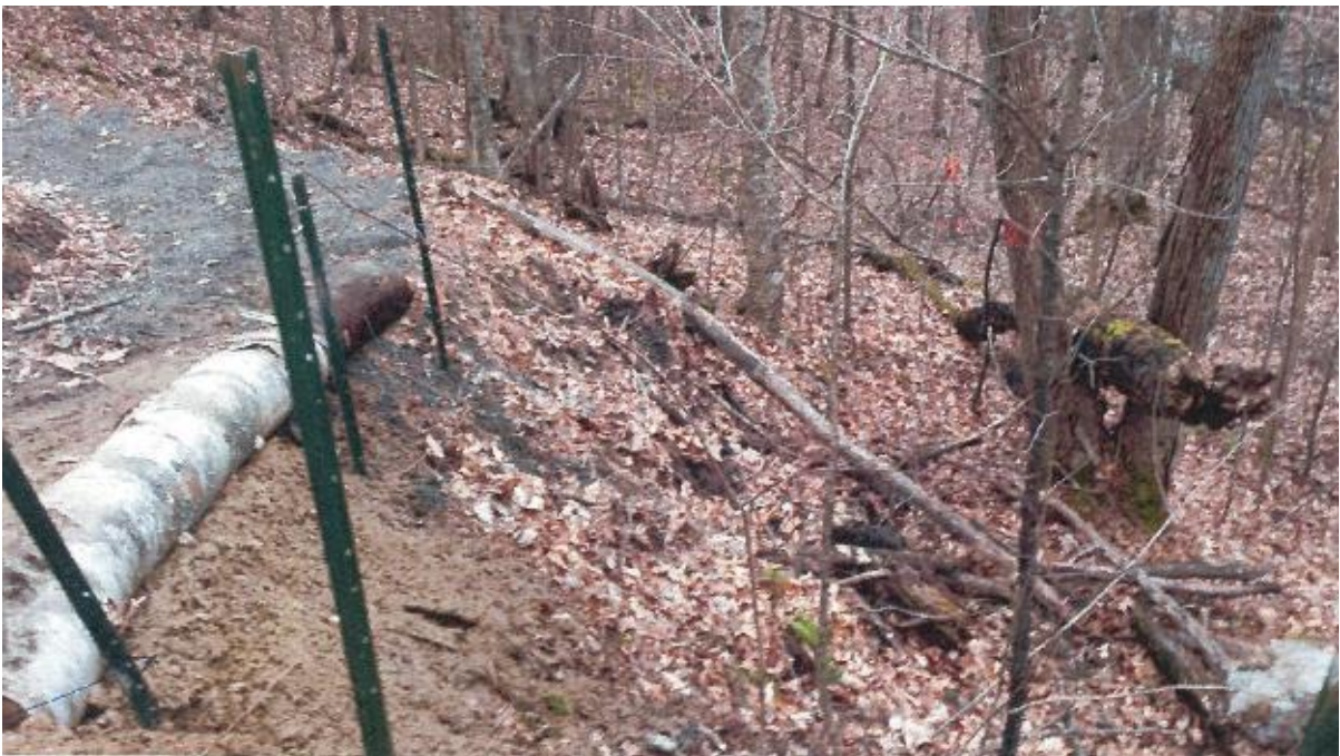
Photo No. 23 – Erosion of slope downhill of pathway. Area approximately 12 m long x 1.5 m to 2 m high.
