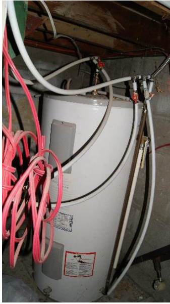
Water heater (basement)
