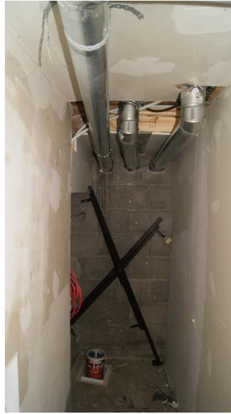
Heating ducts (basement)
