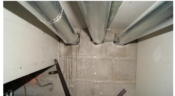
Heating ducts (basement)
