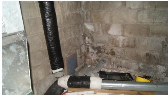
Furnace room (basement)
