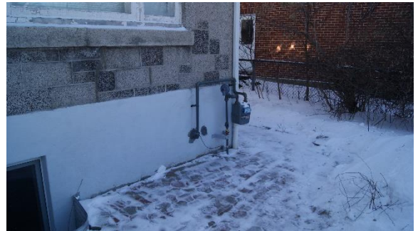
Gas meter (south west)
