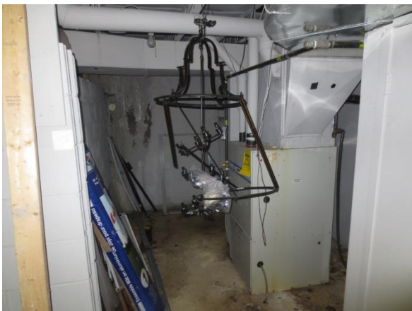
5. View of the natural gas fired furnace located in the basement of the Phase One Property.
