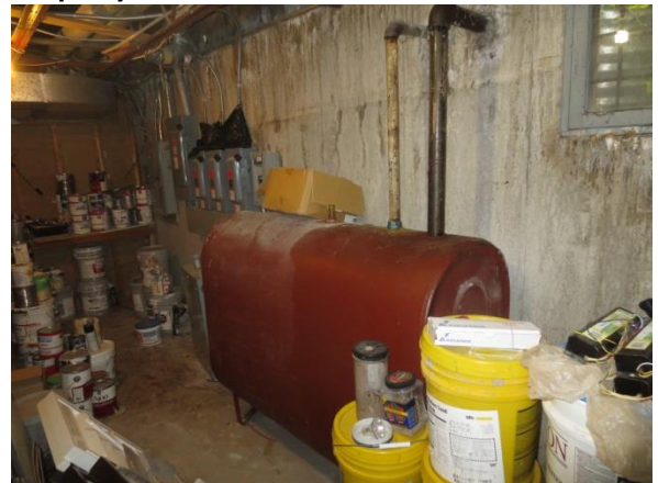
4. View of the fuel oil AST located in the basement of the Phase One Property.
