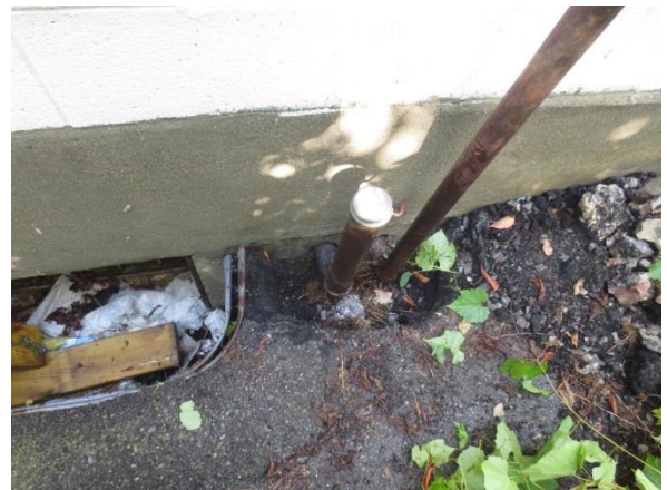
6. View of the vent/fill pipes associated with the fuel oil AST on the southeast exterior of the Phase One Property.
