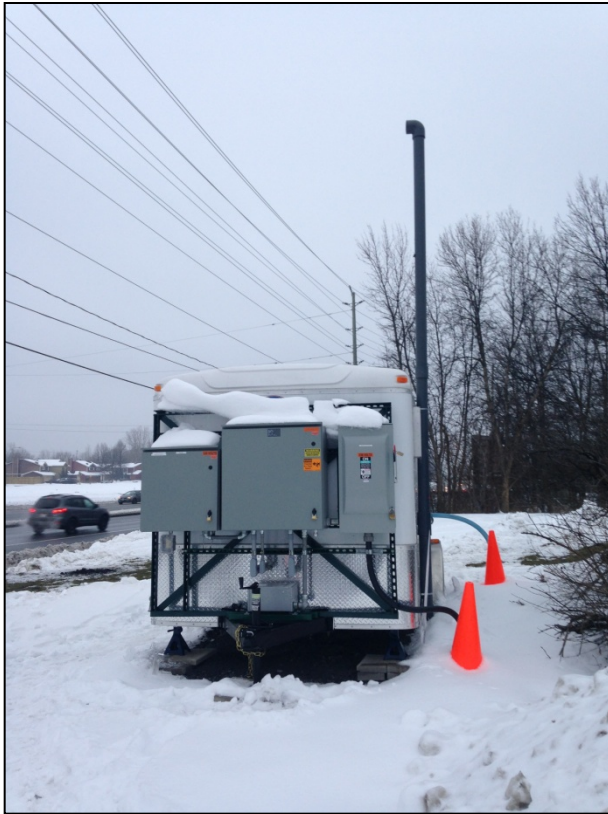
PHOTO 11: Treatment system on-site, looking north.
