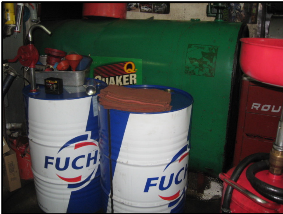
Photograph 8: View of the interior southwest corner of the garage, looking southwest. Photograph illustrates, waste oil storage, staining on floor surface and absorbent material beneath AST.
