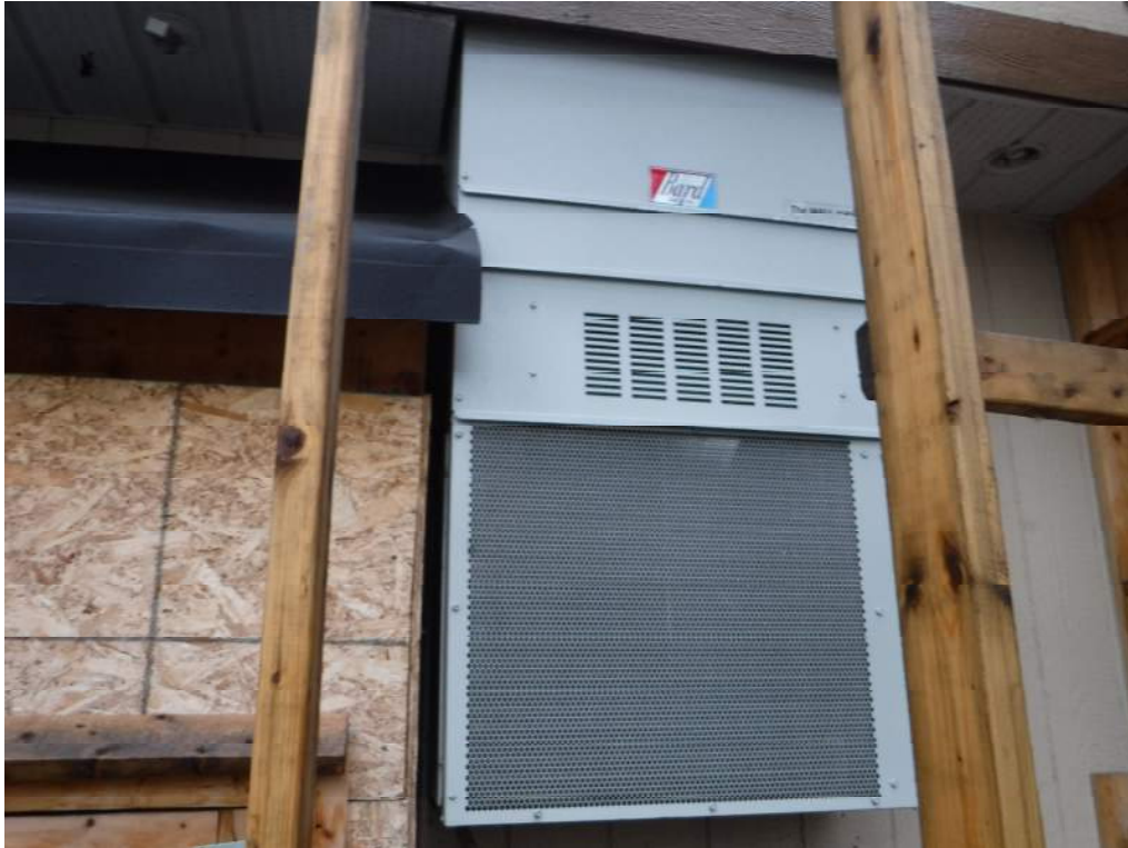
Photograph 7: Air conditioning unit in trailer at Site.
