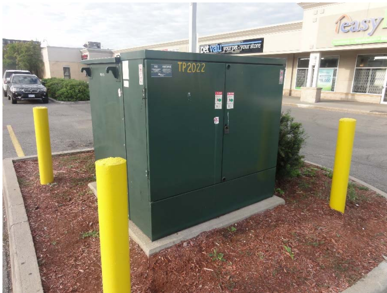
Photo 18 – View of concrete pad mounted transformer on the Subject Property, located southwest of the Site.
