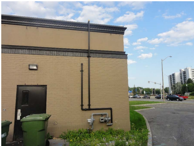
Photo 8 – View of natural gas line for the Site Building, indicating heating and cooling systems are fired by natural gas.
