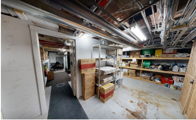
Figure 17 – Stone Residence Basement storage areas. Note painted concrete floor in poor condition, later partition to divide basement spaces, and shelving lining limestone foundation walls.
