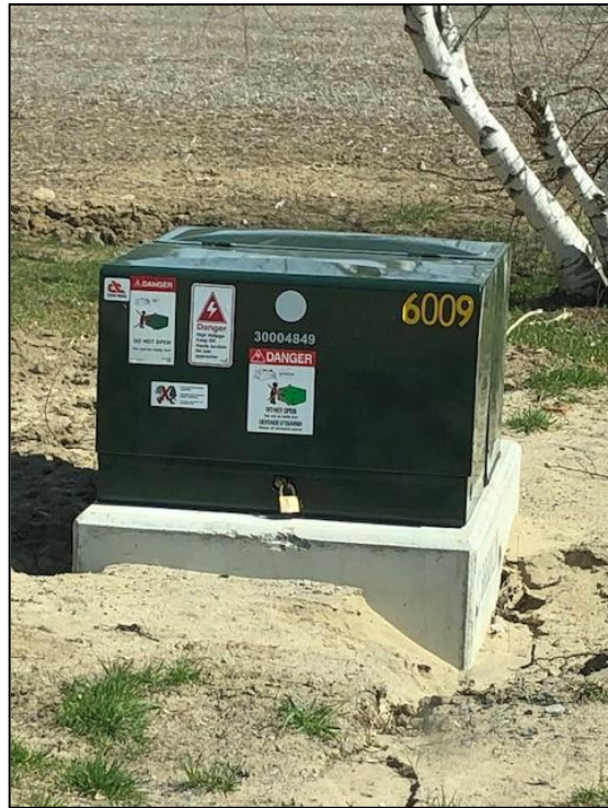
Photograph 3: View of the pad mounted transformer along the western boundary of the subject site.
