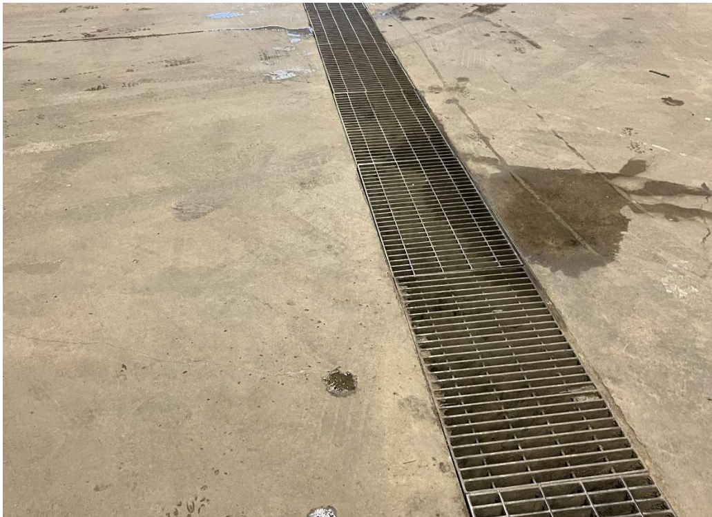
Photograph 4: Trench drain at the center of the service area.
