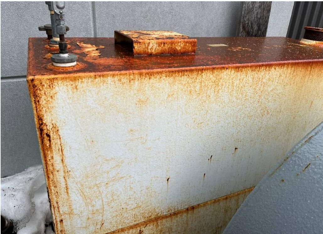
Photograph 6: Waste glycol tank on the exterior of the subject building.
