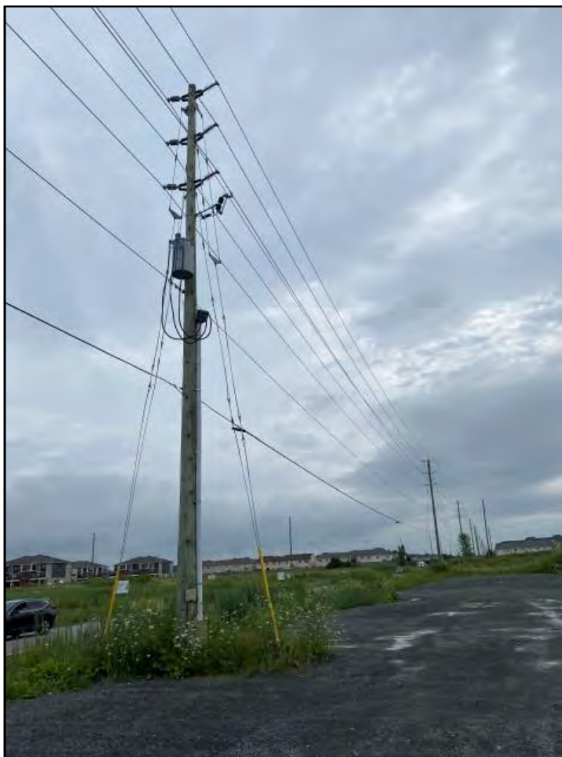
Photograph 3: Looking north at the vehicle entrance to the site from Cambrian Road and a pole mounted transformer beyond the north property boundary.
