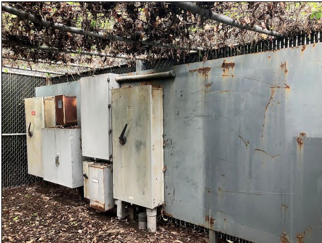
Photograph 6: View of natural gas compressor, looking to the north.
