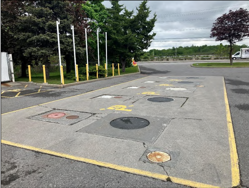
Photograph 3: View of UST nest, looking to the east.
