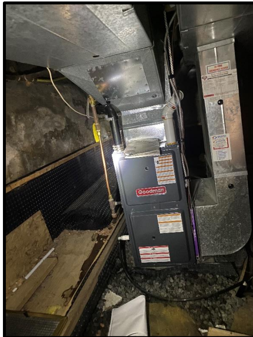
Photograph 8: View of the natural gas forced air furnace inside the 339 Roosevelt Avenue dwelling.
