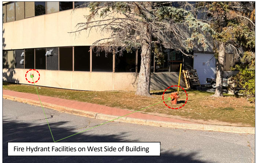
Exhibit 5-2: Emergency Water Sources on West Side of Building
