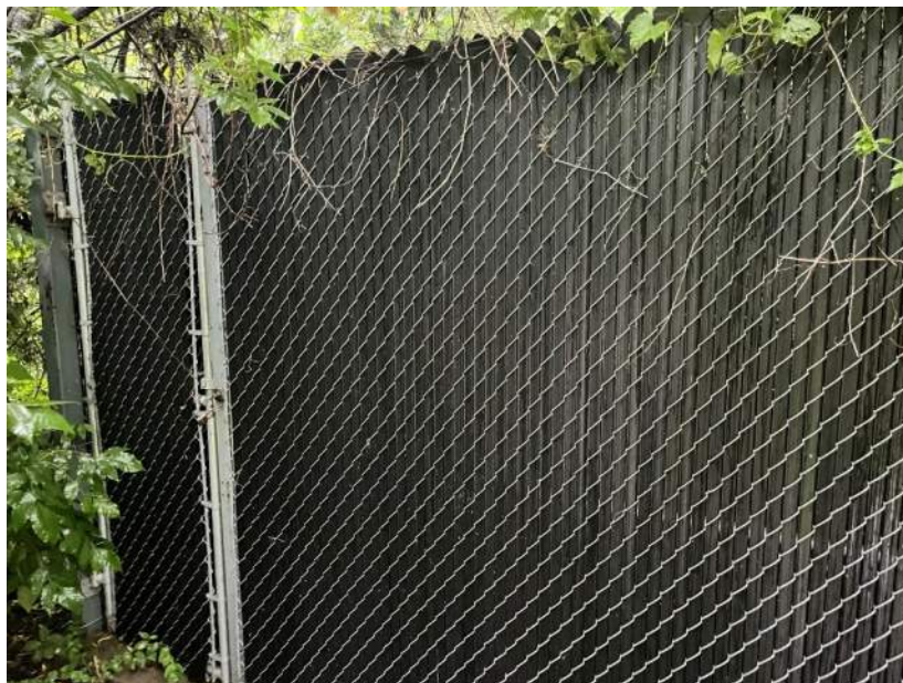
Photograph 4: Existing 3 rd party natural gas compressor enclosure to remain. Direction: Northwest
