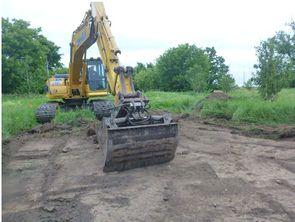
Image 46: Komatsu PC 200 LC tracked excavator with a 1.6 m wide smooth bucket completing MTR in Operation 2, view north.
