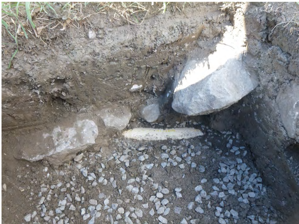
Image 34: Gravel fill (Lot 8) and PVC pipe observed in northeast corner of test unit 3S 39E, view north.
