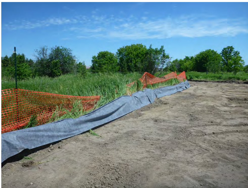
Image 47: Geotextile fabric placed along exposed profile adjacent to City of Ottawa owned land in Operation 2, view north.
