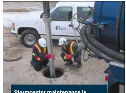
Stormceptor maintenance is performed at grade with a standard vacuum truck
