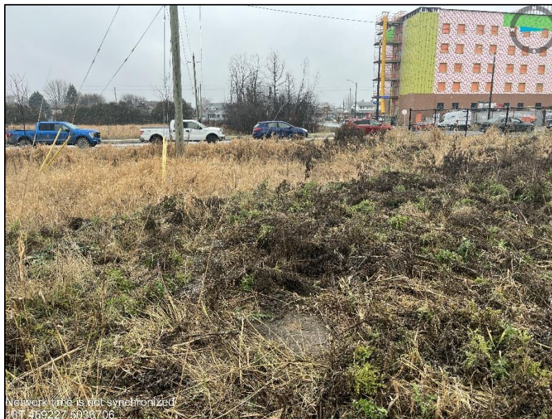
Municipal storm sewer manhole observed in the southeast portion of the Site
