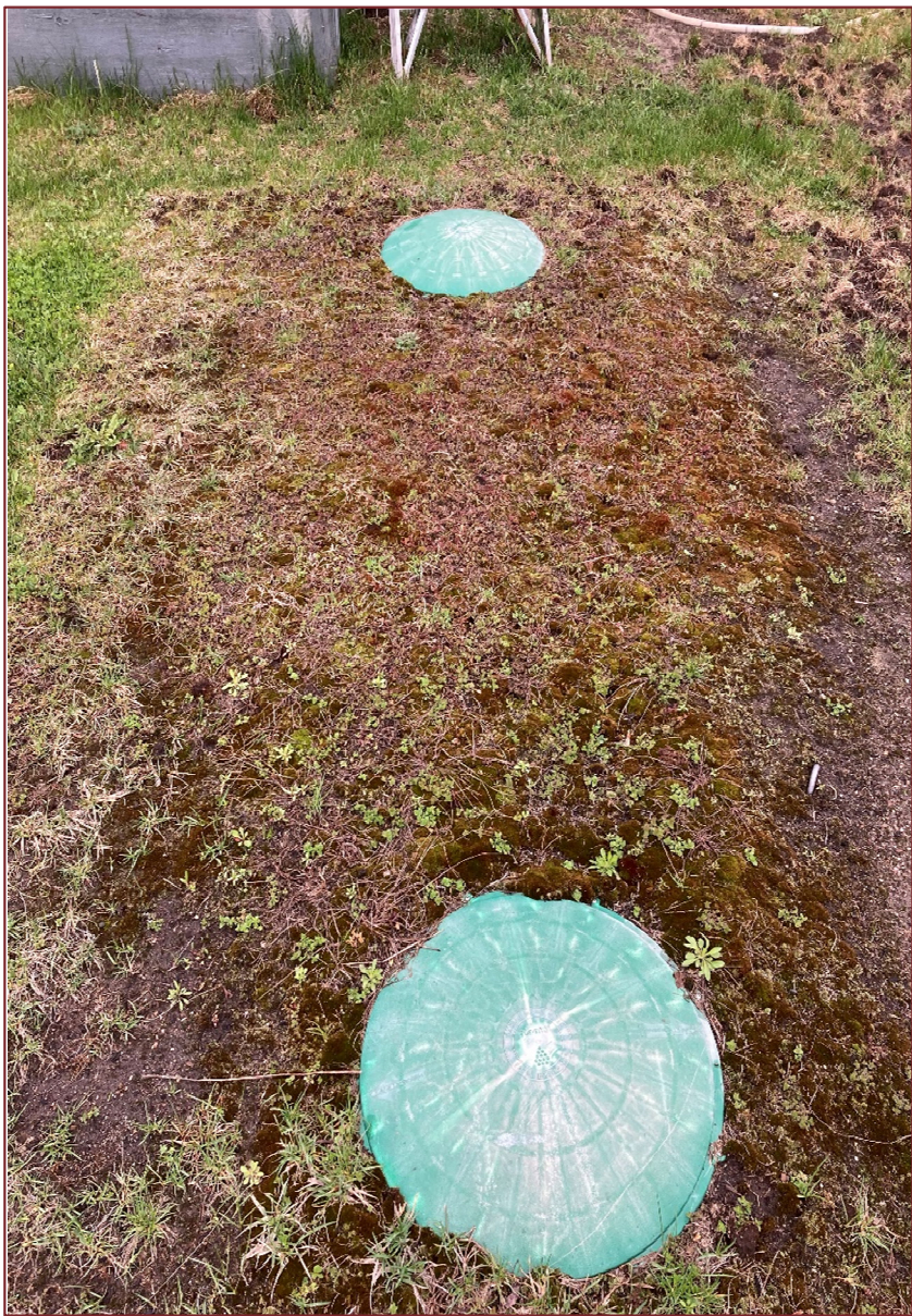
Photograph 31: Septic Tank for CACE Construction portable.
