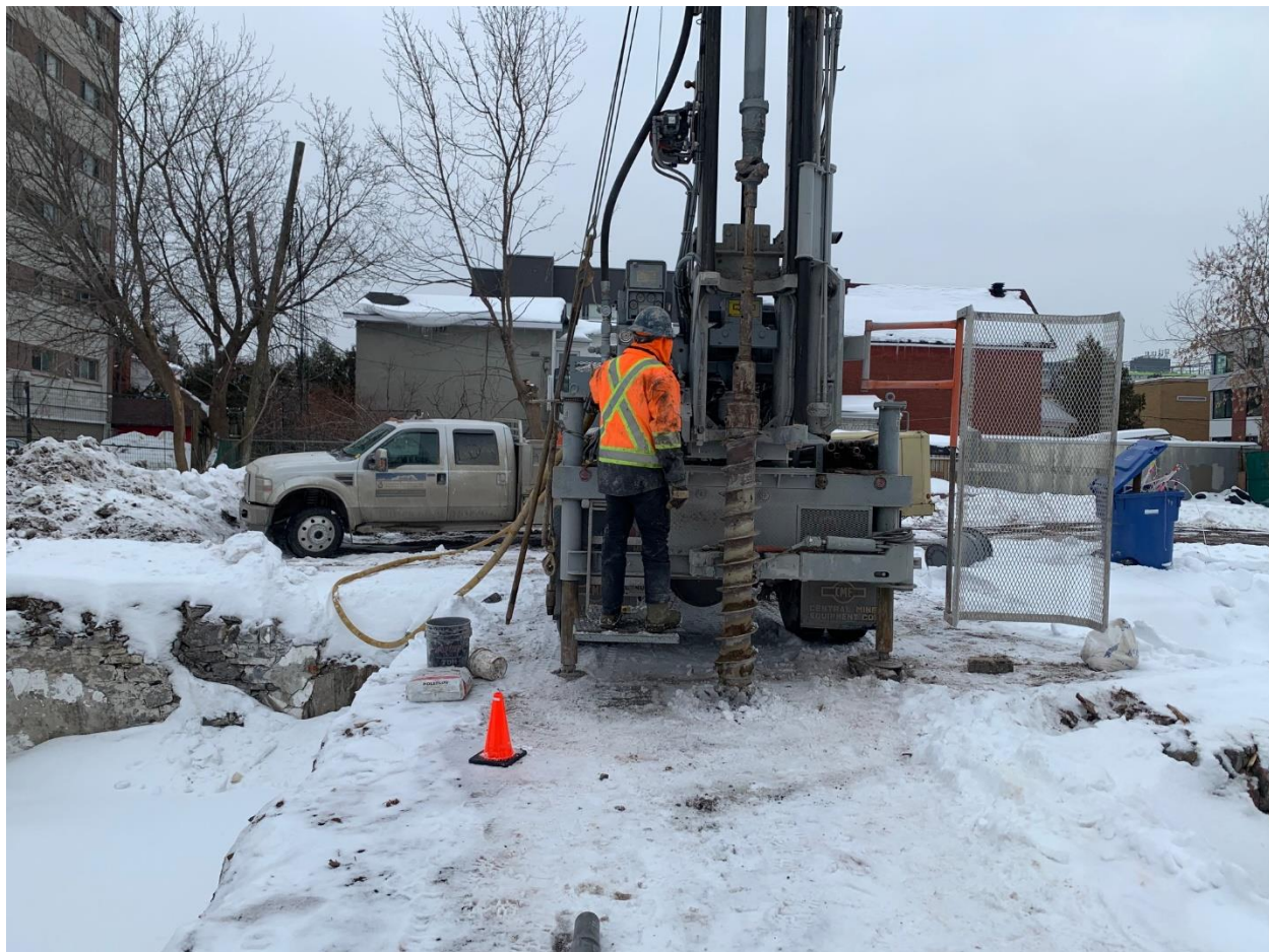
Image 2 – Monitoring Well 1, facing east (later decommissioned)
