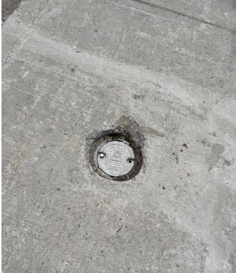
Image 8 – EX-MW6 offsite monitoring well
