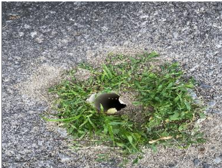
Photo 8 – Groundwater monitoring well (damaged) identified along the east boundary of the Phase One Property. Fill material of unknown quality identified here (PCA).
