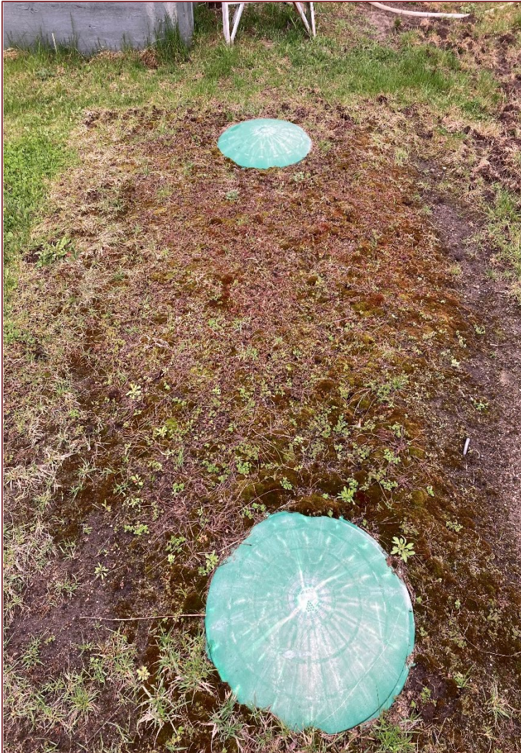
Photograph 31: Septic Tank for CACE Construction portable.
