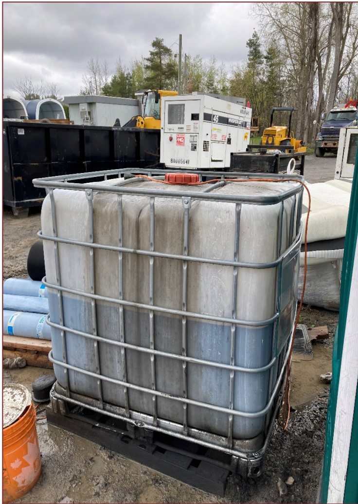
Photograph 27: Tote containing waste oils from CACE construction.
