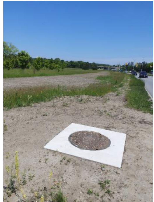
Photograph 28: View of newly installed manhole facing north, located across Riverside Drive, west of Lot D.
