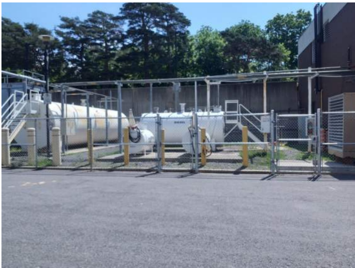
Photograph 43: Diesel storage tanks associated with hospital operations, facing east.
