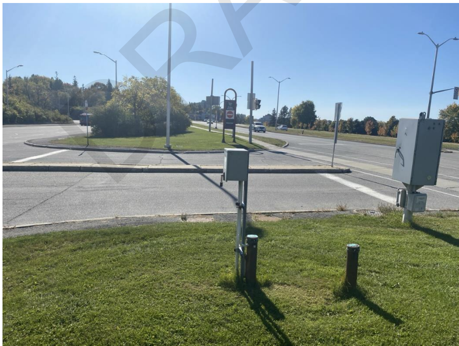
Image 2: Utilities at south limit of north Study Area fronted by bus lane. Facing south.
