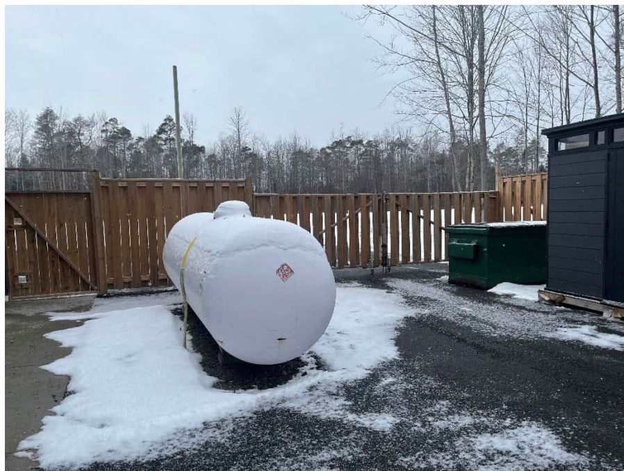
Photo 16: Large propane tank located to the north of the main building. No noted secondary containment.
