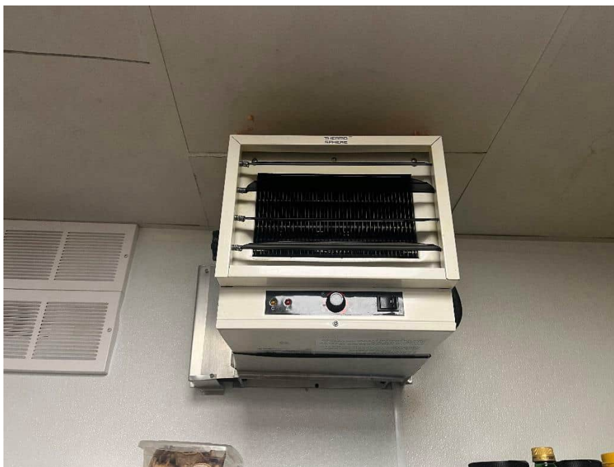
Photo 11: Suspended heater in kitchen trailer.
