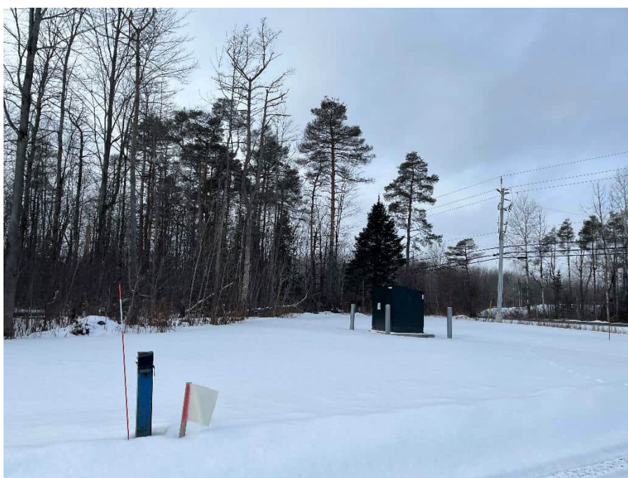
Photo 30: Monitoring well and transformer adjacent to Franktown Road, nearest from entry of Site driveway.
