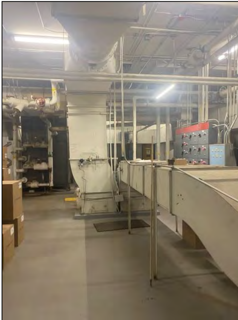
Photograph 11: View of a mechanical room on the north side of the subject building (room 301).
