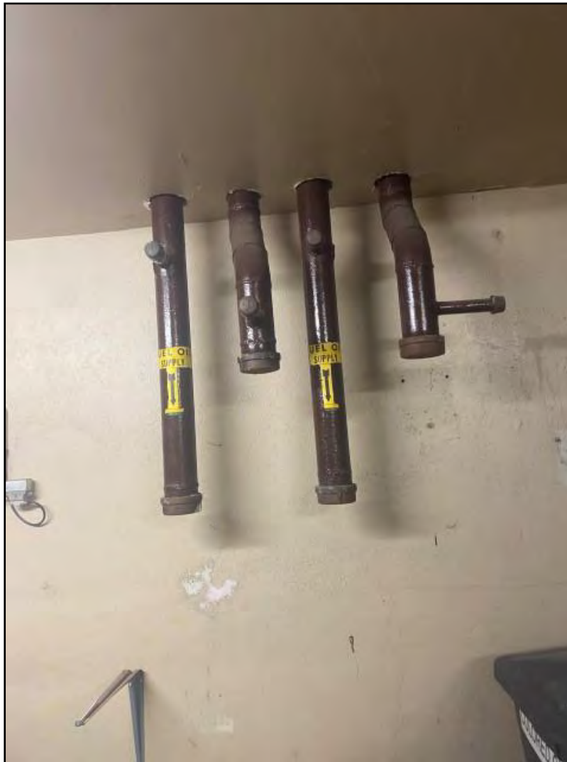
Photograph 14: View of former fuel oil pipes in room B001.
