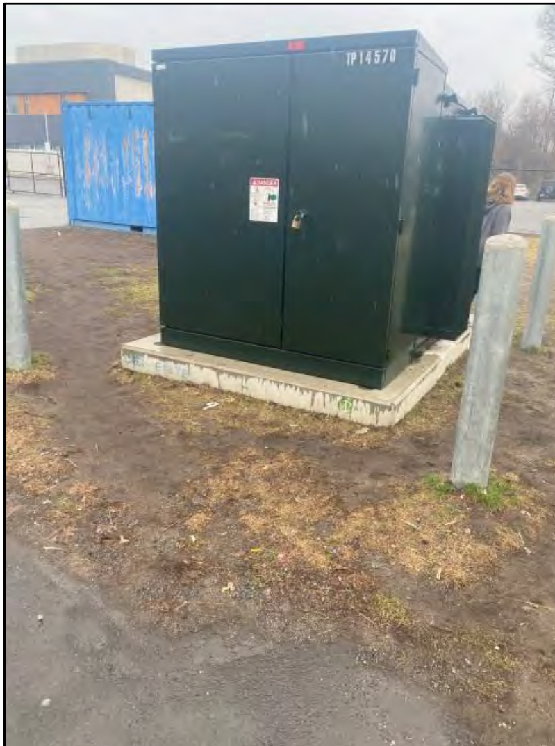
Photograph 3: View of the ground mounted transformer on the south-west side of the building.
