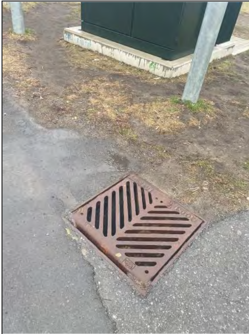
Photograph 4: View of a stormwater catch basin on the south-west side of the building.
