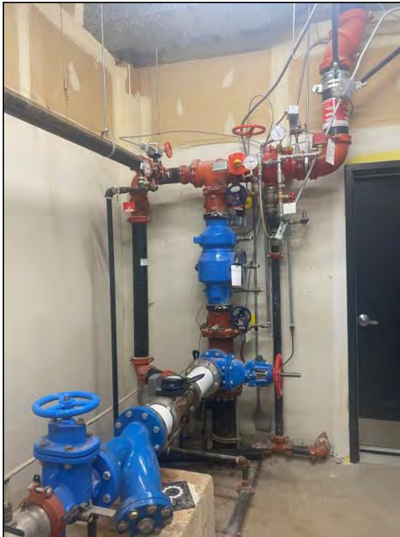
Photograph 12: View of the backflow preventor on the south-east side of the school (adjacent to entrance D1).
