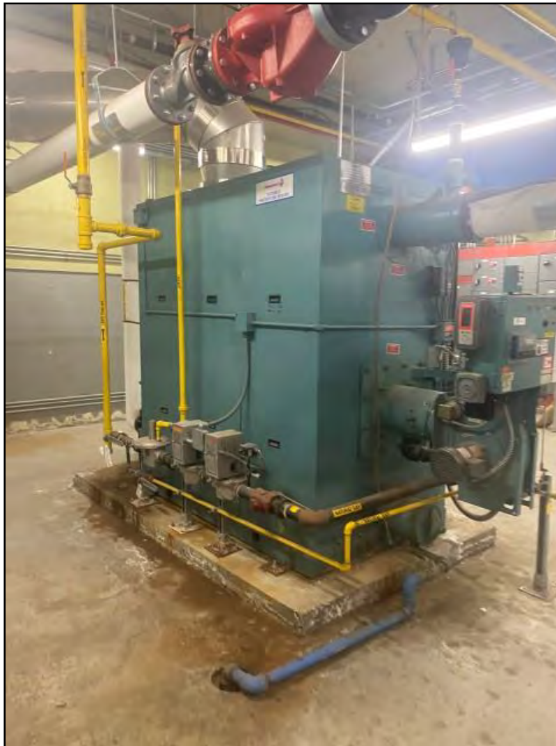
Photograph 15: View of the boiler room (B006). Minor staining from rust/water is in view.
