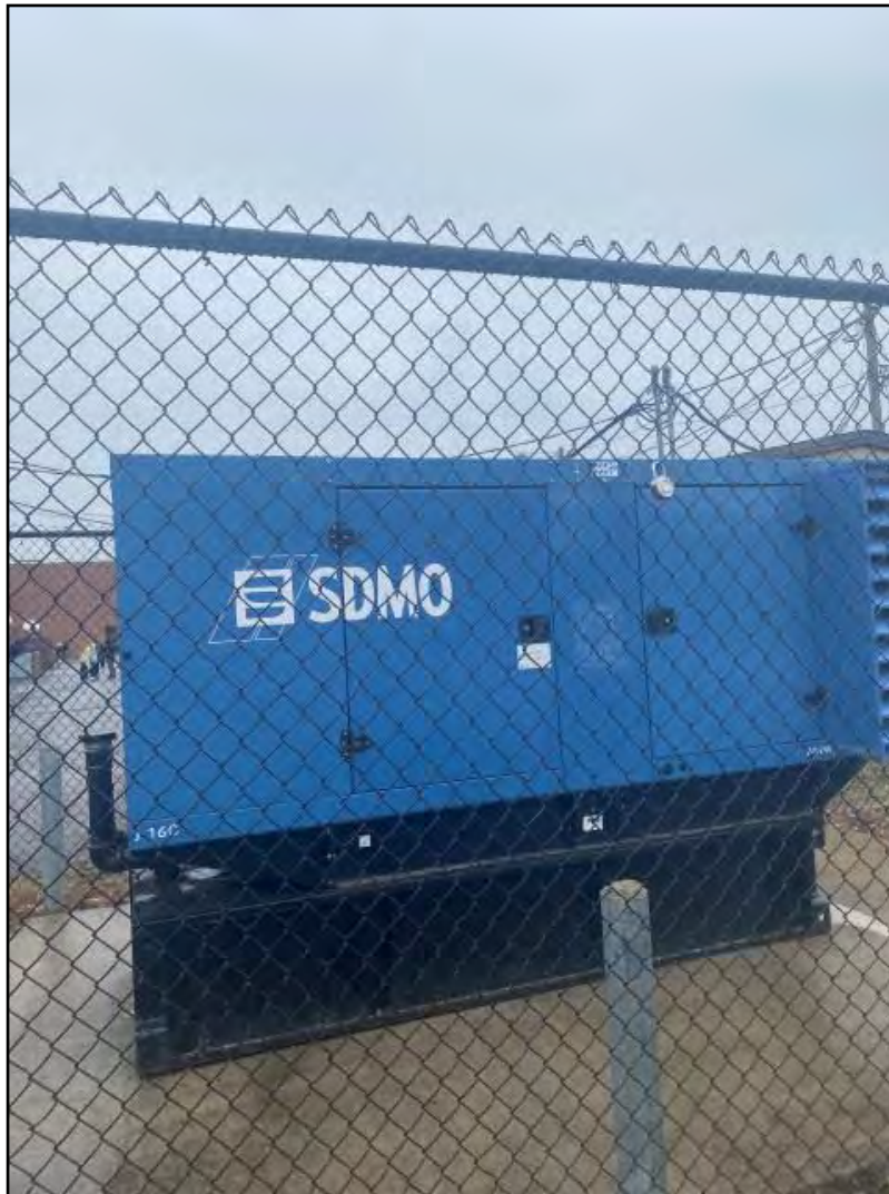
Photograph 6: View of the diesel-powered generator on the exterior west side of the building.
